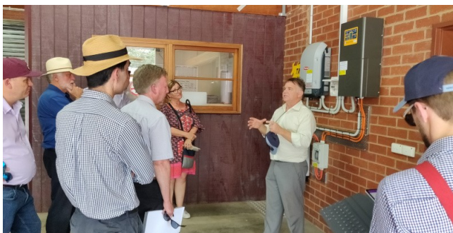
Matt Charles-Jones shows the legislative committee the solar and battery system at the Yackandandah CFA station
