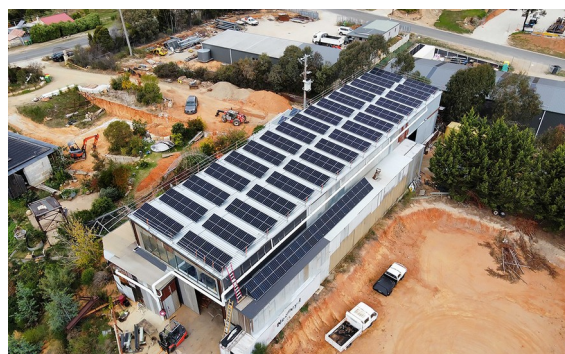
The 65 kW of solar panels on the roof of the old sawmill that are part of the Yack01 community battery installation.
