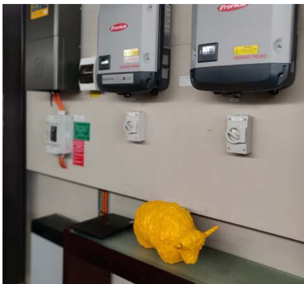
TRY's Golden Yak below the Fronius inverters at the launch of the Virtual Power Plant in the Yack Public Hall
