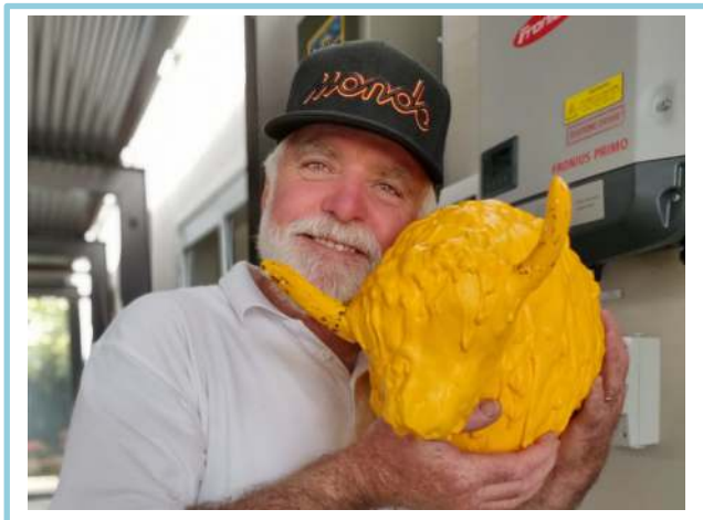
Denis Ginnivan and golden yak, standing in front of the Fronius inverter and 13 kWh of batteries at the Virtual Power Plant launch, Yack Public Hall
