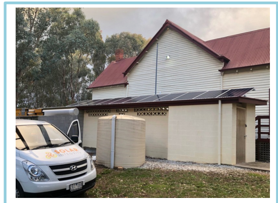
Osbornes Flat Hall during the recent installation of its new solar system
